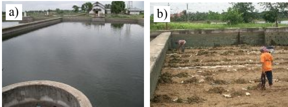
Photo 1. Water purification plant, a) Slow sand filtration Pond b) Cleaning up of clogged pond
