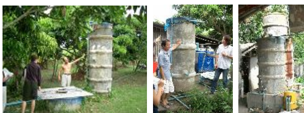
Photo 6 Filtration tower in house garden for treatment of groundwater
