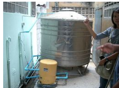
Photo 4 water storage tank and feed pump in household
